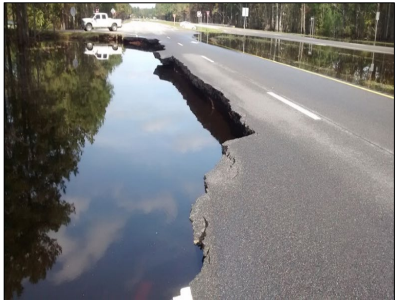
Figure 1: Large pavement failure in eastbound US 74 following Hurricane Matthew, October 2016
