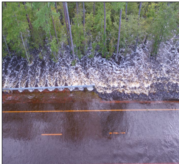
Figure 14: Extensive flooding following Hurricane Florence, September 2018
