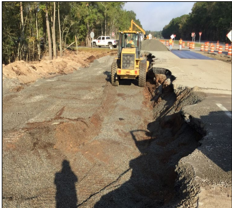
Figure 15: Repair to shoulder after Hurricane Matthew, October 2016
