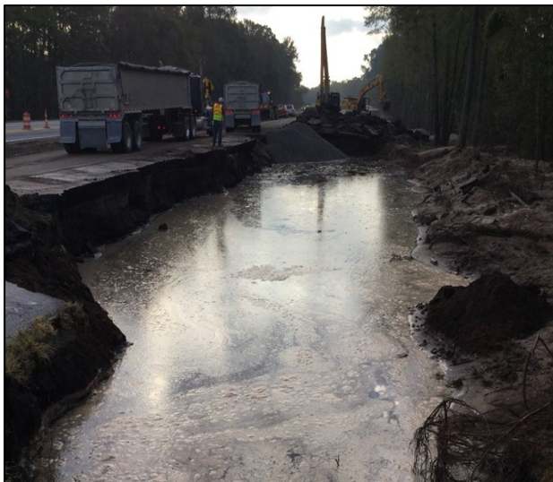
Figure 4: Corridor damage and repairs after Hurricane Matthew, October 2016
